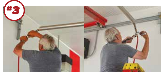
#3 By hand, attach the new hose threading into the connection point at the boom, then tighten with wrenches.
